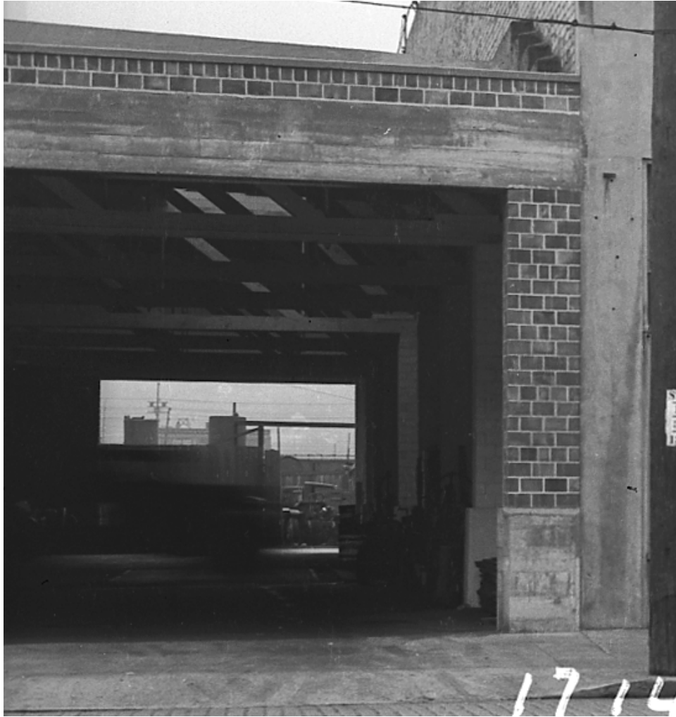
Detail of far south portion of west elevation, 1937 tax assessor photo of adjacent building, showing partial interior of the subject building, including roof trusses.
