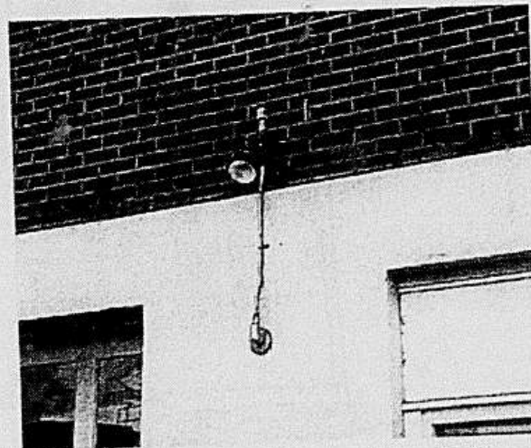
Photo 4.2.46 Building 29 added exterior floodlights
