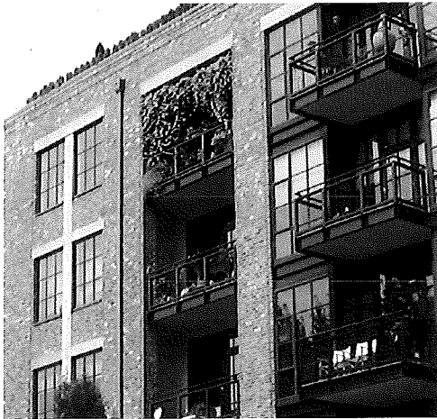
Brick masonry and metal balconies Brick masonry can be a beautiful, durable, and regionally appropriate material for a building facade; balconies clad in metal like those seen here are preferred at Yesler Terrace. (Photo: GGLO)
