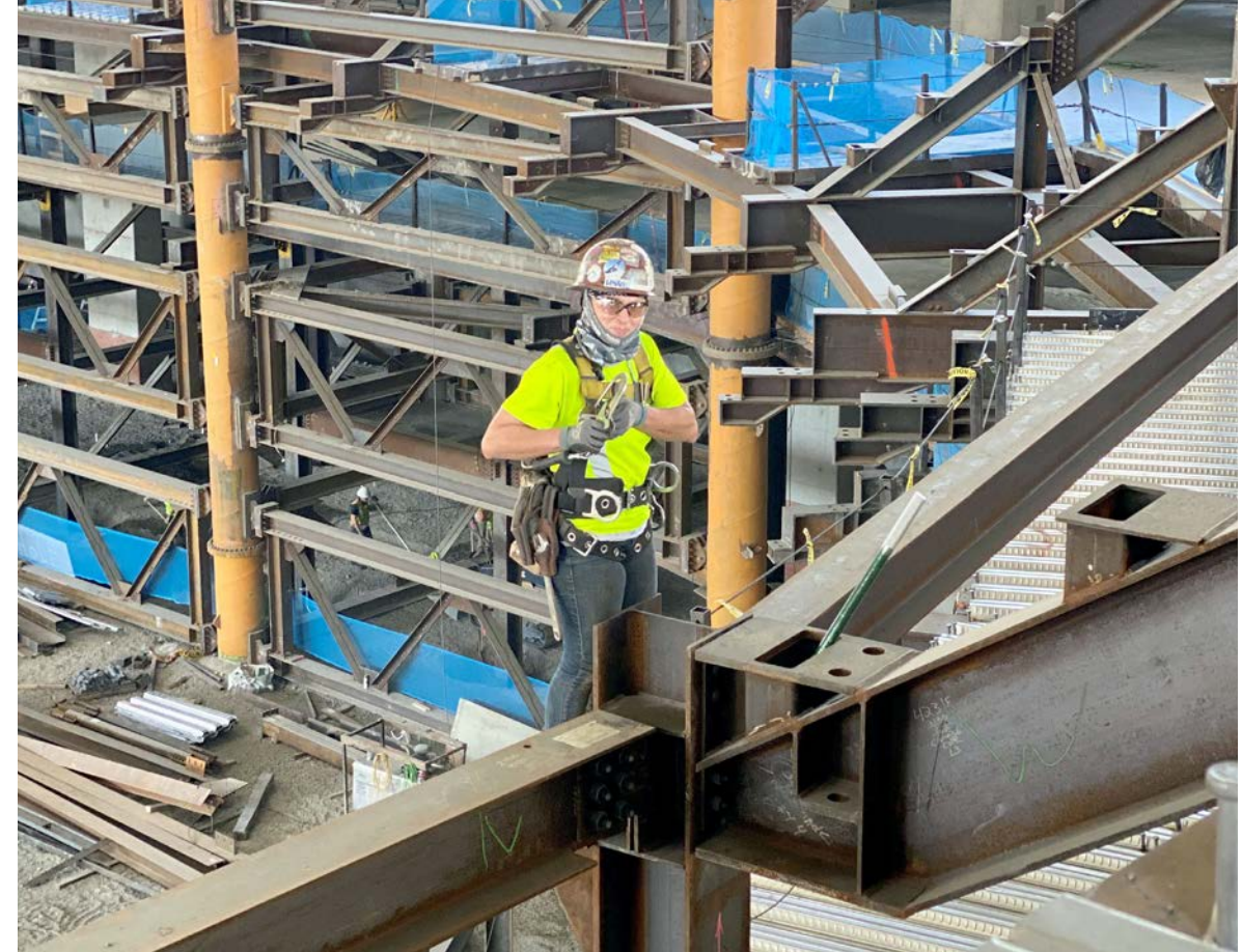
Jessica worked as an ironworker apprentice for Danny’s Construction and Farwest Steel on the Climate Pledge Arena for over a year, earning more than $123,000, plus benefits. Jessica completed the TRAC pre-apprenticeship program, which provides basic construction and job-skill training for incarcerated women. Jessica’s work on the Arena helped her gain the experience needed to advance in her apprenticeship — she’s now close to becoming a journey worker! Photo courtesy of the TRAC pre-apprenticeship program.
