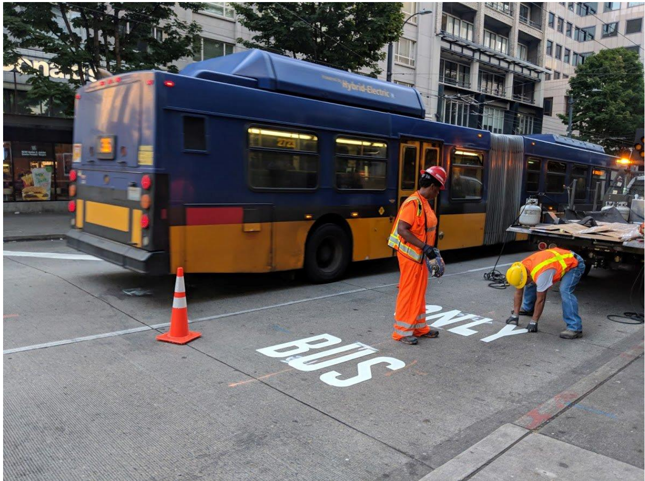
Crews working to install red bus lanes to keep transit moving through critical areas around town
