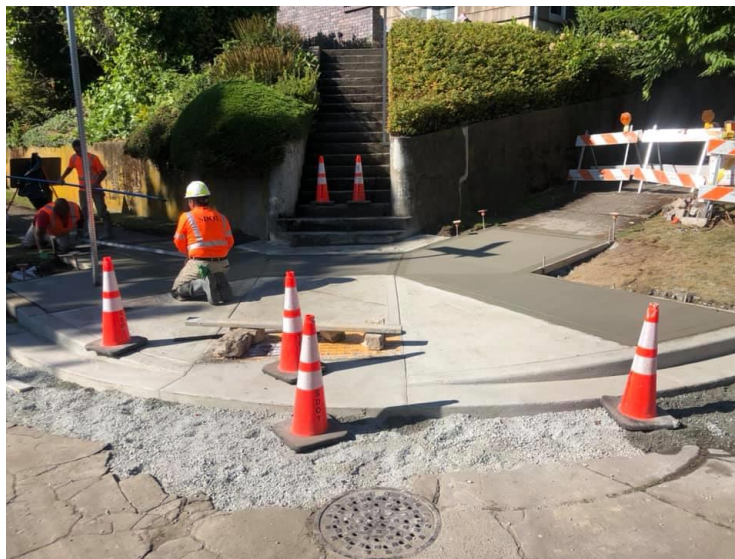
In 2019, crews worked hard to exceed the planned accomplishment, building curb ramps that are compliant with ADA standards through the Customer Service Request process.
