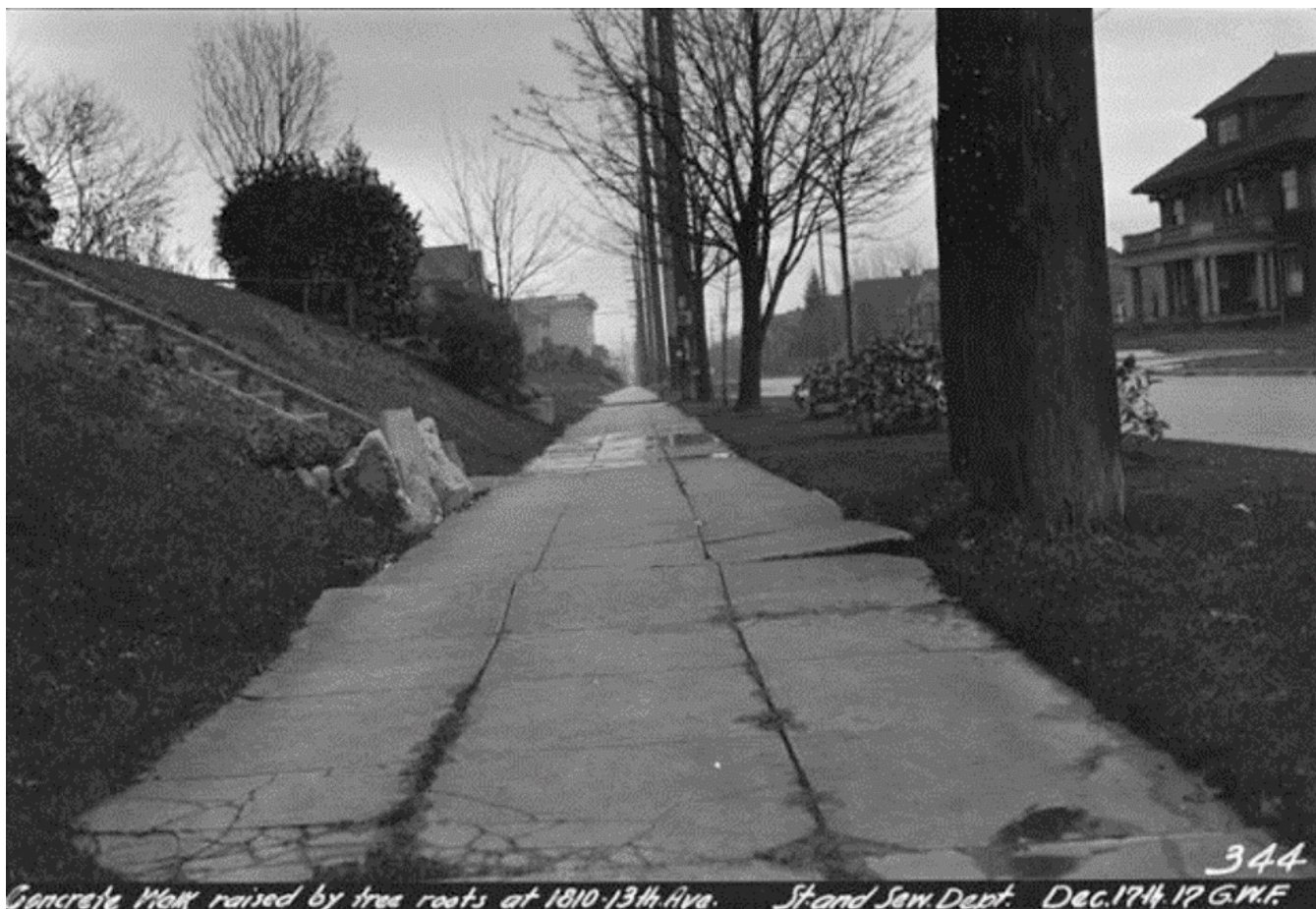
A Seattle sidewalk damaged from tree roots (1917)
