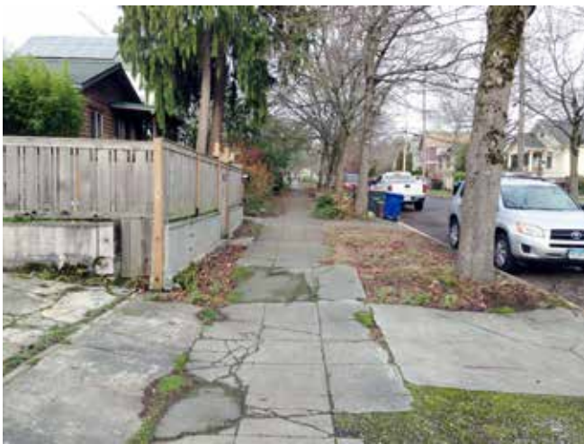
A damaged sidewalk prior to repair and after
