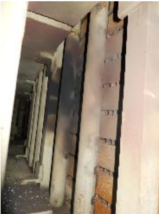
Unit 53: Note slag from damage to core
