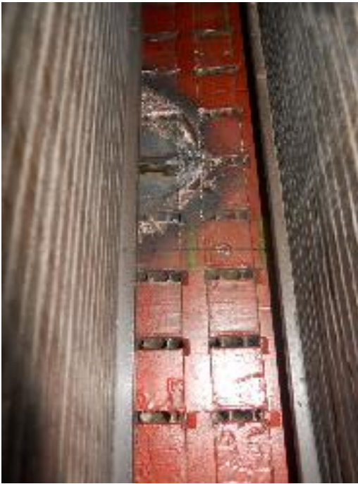
Damage to Unit 53
