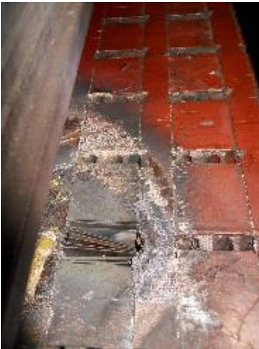
Unit 53: Separation of laminations
