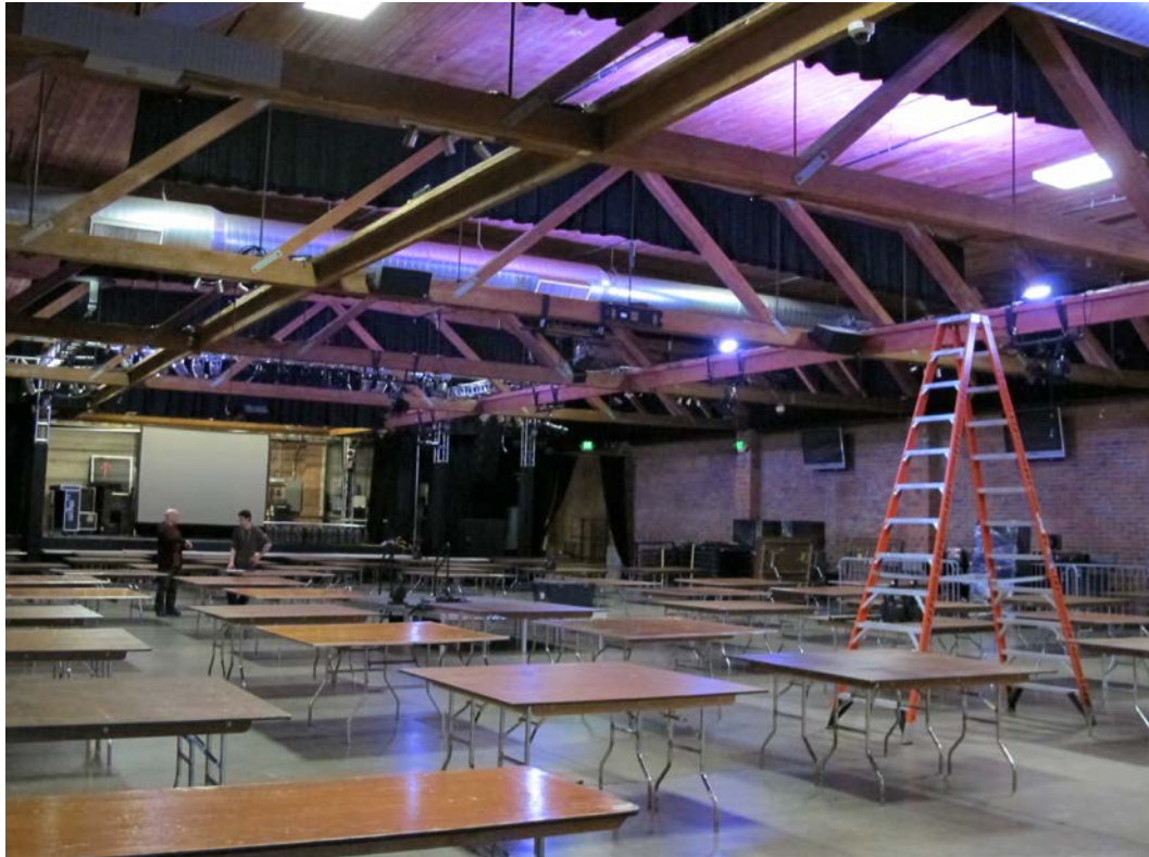
Interior of live music venue portion of space. Note timber and steel cable components of roof trusses.
