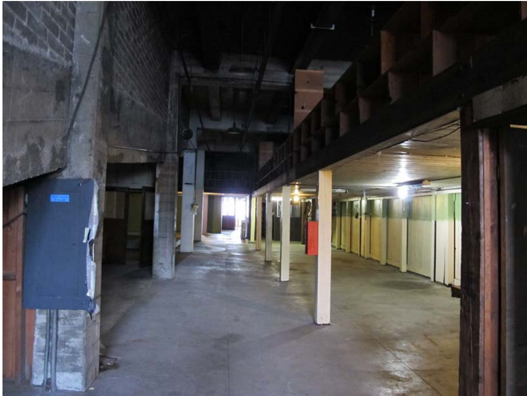
First floor, southern half of building A. Auto/truck ramp is at left, on other side of masonry wall. The purpose of the openings along the wall at right could not be discerned, but may have been warehouse-related storage spaces.
