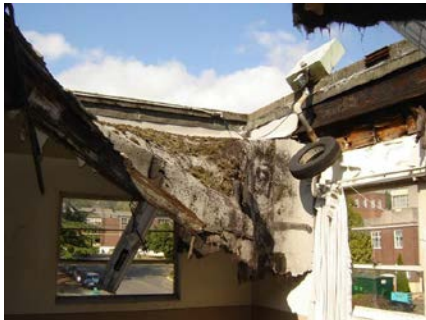
A deteriorating building at Magnuson Park
