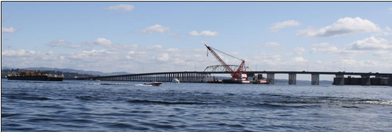
View of construction barges on the north side of SR 520, near Madison Park.
